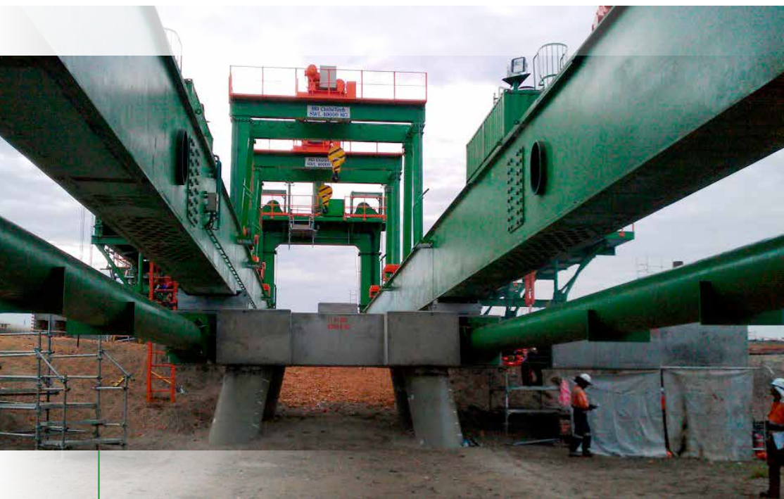
The substructure of an LNG jetty in Port Moresby, Papua New Guinea
